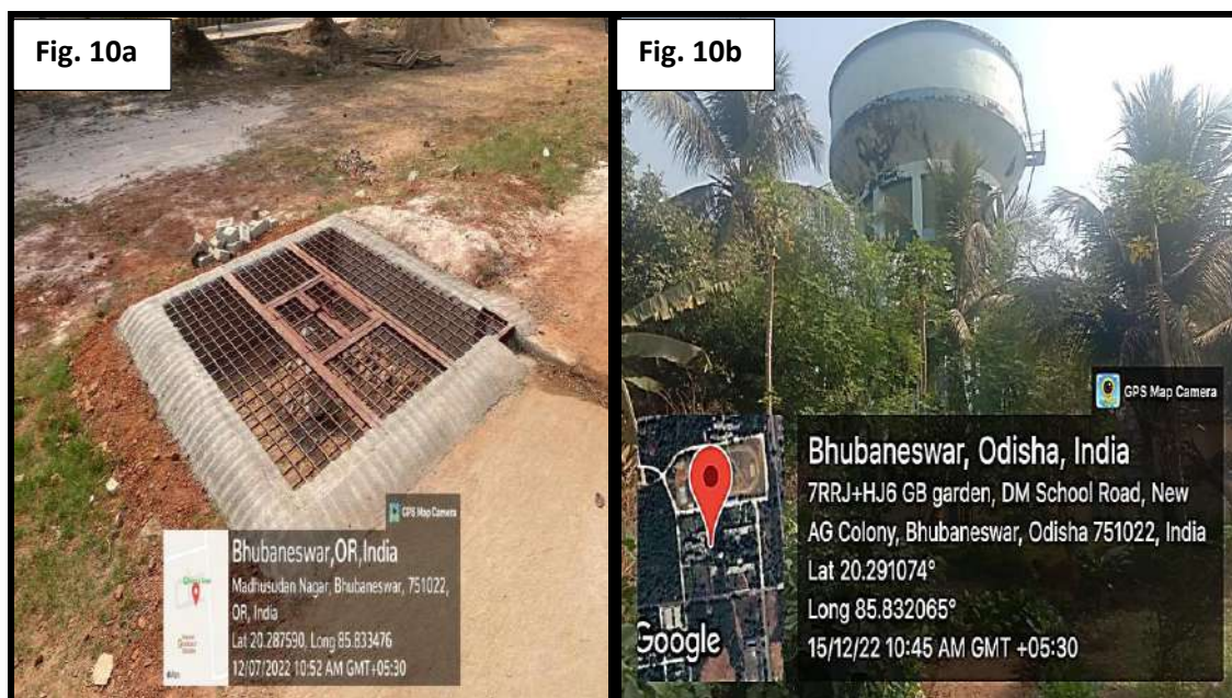
Fig. 10a – Borewell near D.M.School Cycle Stand; Fig. 10b – Photograph of overhead tank which supplies water in the Institute
